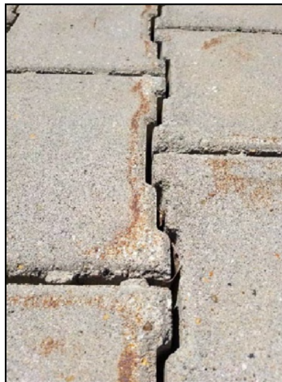
Rust marks from steel snow blades
