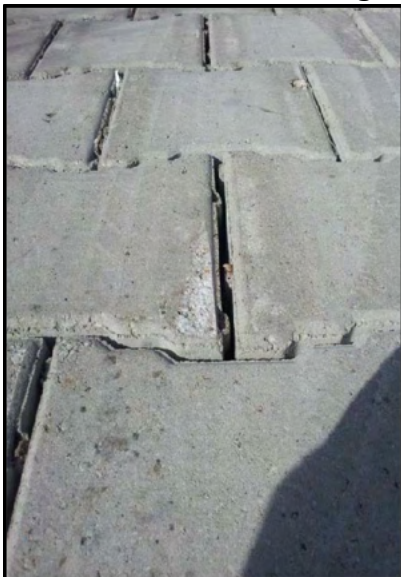
Steel Snow Plow Damage
