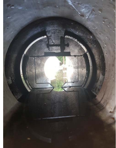
V-notched weir mounted inside 8-inch steel drain pipe
