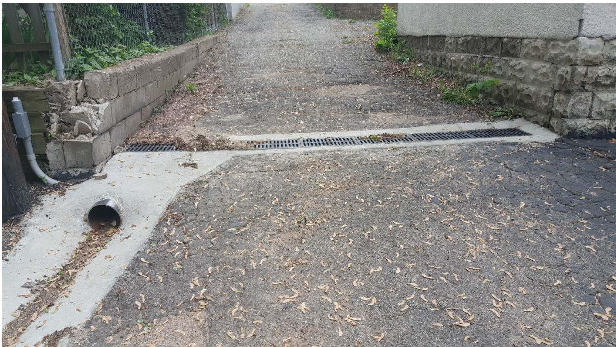
Trench drain with 8-inch steel drain pipe and flow data logger, 2017
