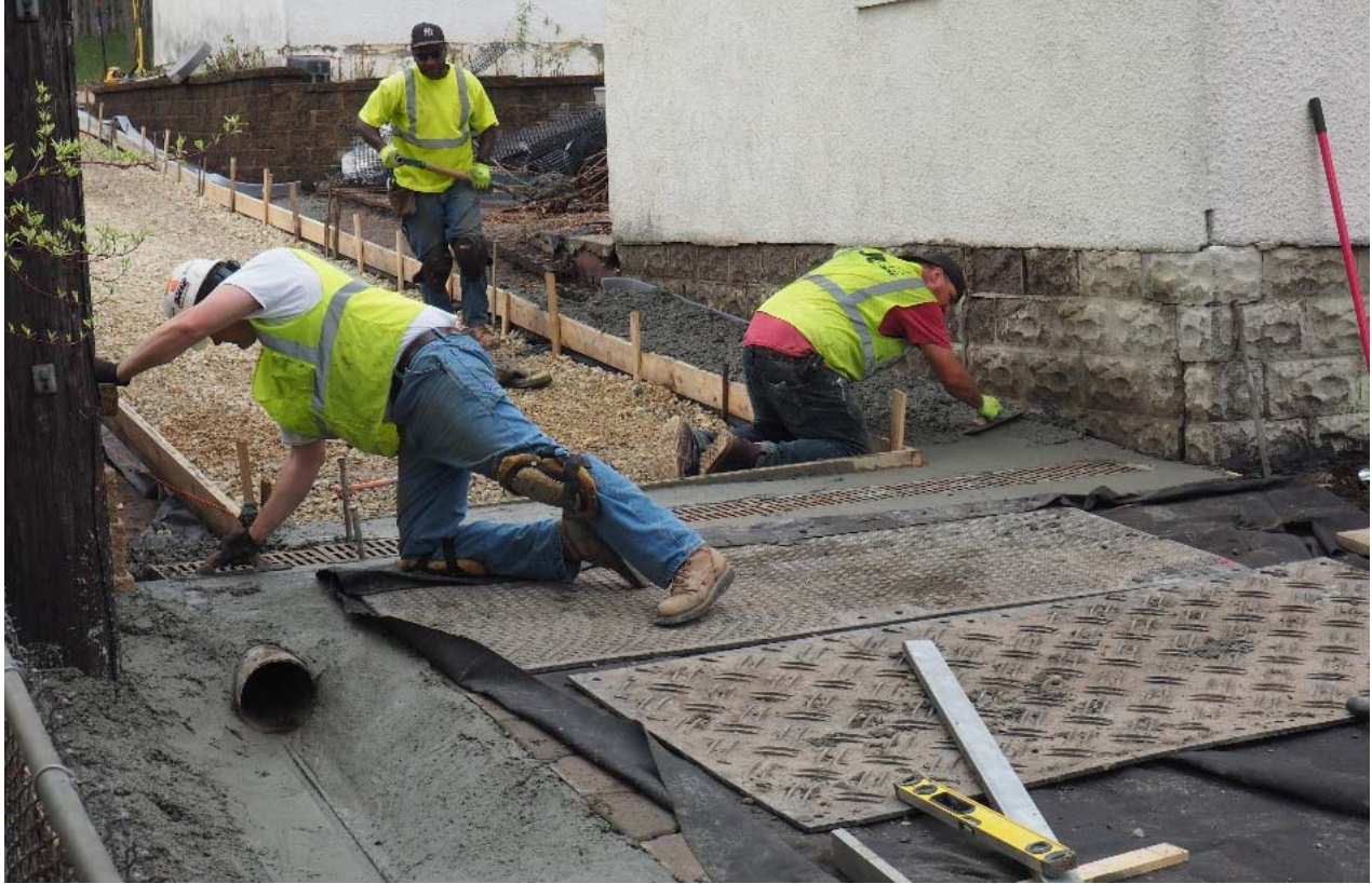
Concrete pour and trench drain / 8-inch steel drain pipe and re-installation in same location as 2017
