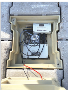
The INFIL-Tracker is a below pavement sensor.
